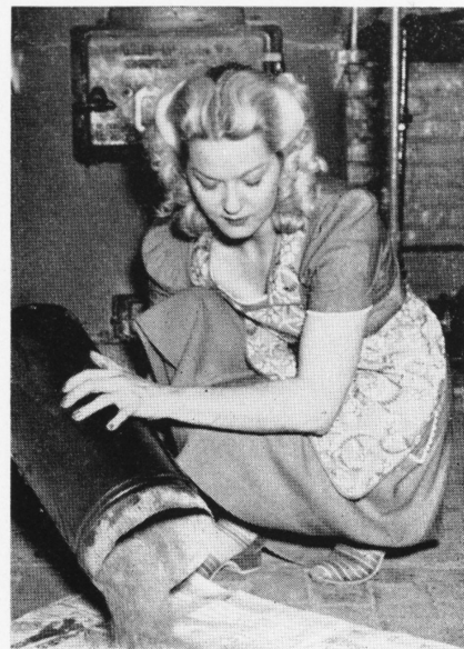
This home manager is getting after the heater smoke pipe in her cellar and getting all the soot and ash out of it. This will help a lot to give the heater a better draft when the bitter cold days come next winter.
